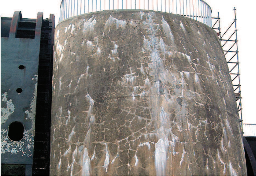
Figure 1: ASR affected concrete construction showing extensive cracks and the escape of the alkali-silica gel. As the gel reacts with the atmosphere, a characteristic white carbonated efflorescence remains on the surface of the construction.
